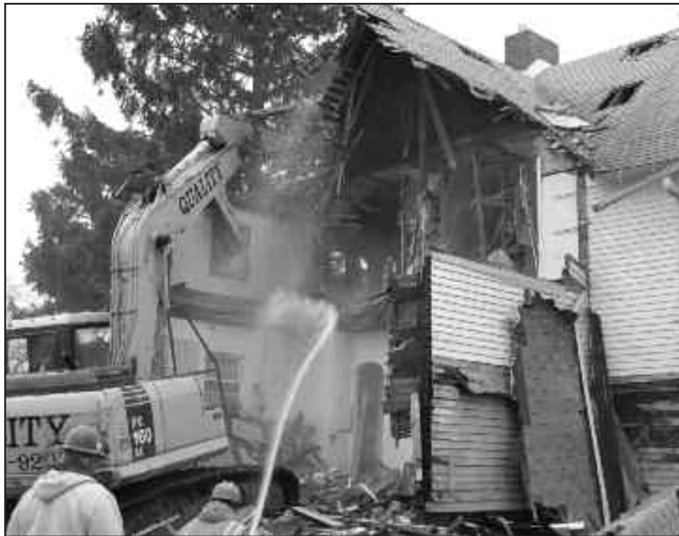
Water is sprayed on the more than 100-year old Parsonage Victorian House, 6049 N. Northcott Ave. to reduce dust during demolition. Several days earlier, the Chicago Fire Department conducted simulated fire training exercises in the building.
